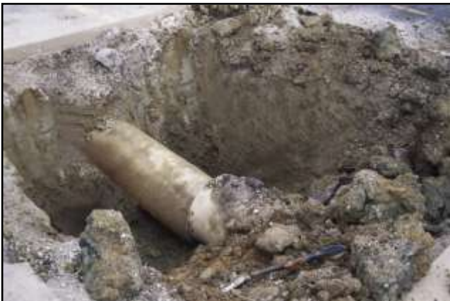
Defect 3: A collapsed pipe.
