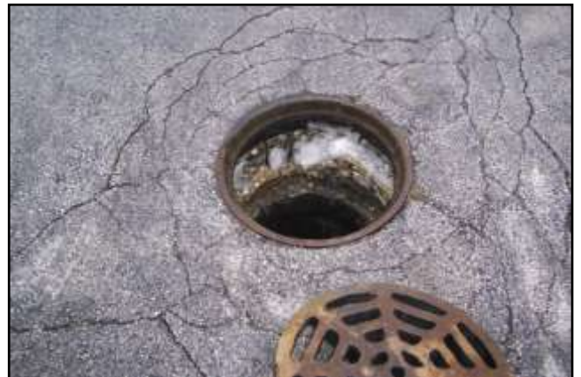
Defect 4: Frost heave has caused this basin to shift.
